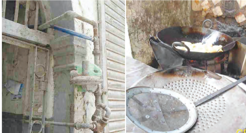
A restaurant was being run through an illegal connection
